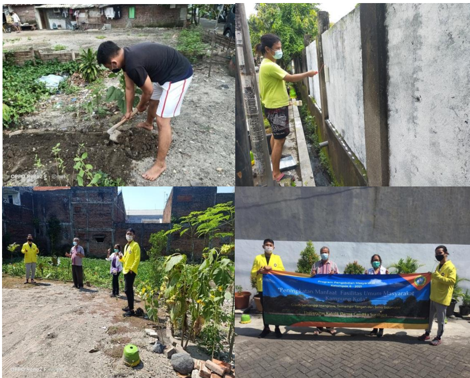
The pictures above show a series of activities in KKN-PM location in Semampir Tengah 4-A/RT 2. Our community service works include repainting the alley wall, removing clinging vines, and planting sunflowers in vacant lots.
